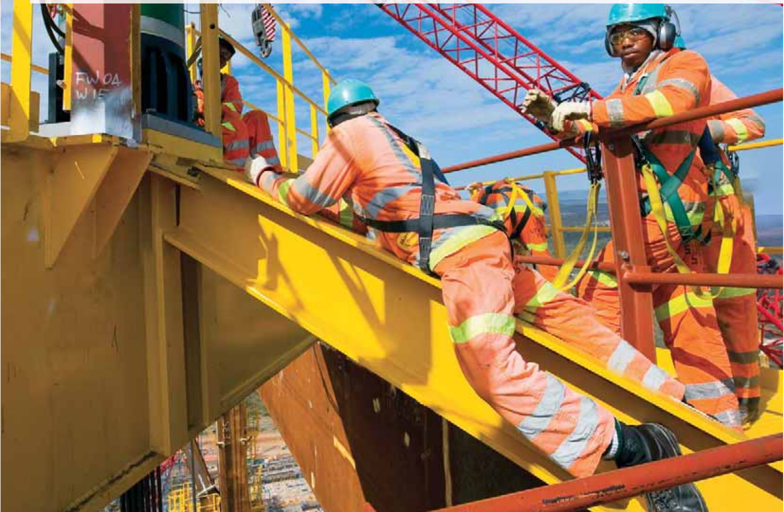
Medupi power station boiler mainframe
