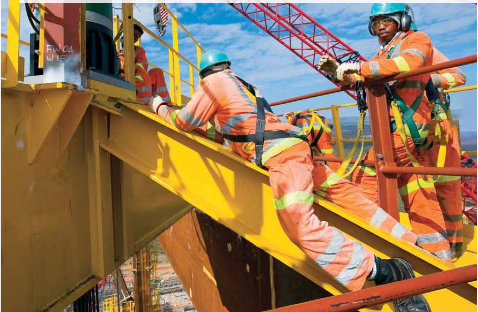
Medupi power station boiler mainframe
